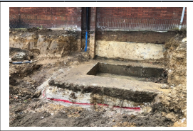
24th May - Uncovering foundations from the Forum within the footprint of the MSCP
