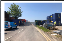
15th May - Offices and welfare facilities in place on the West of the site
