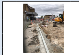
10th July - New kerb line installed for the taxi rank area in front of the station
