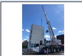
31st July - Final lifts being carried out for the Eastern stair core
