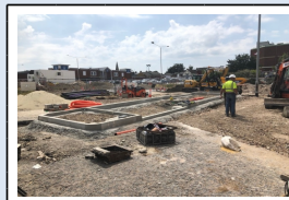
4th July - Kerbing installed for the new pedestrian crossing island at the end of Dover Street
