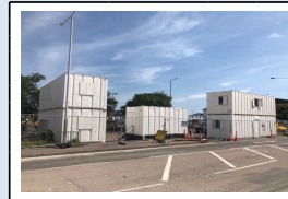
15th June - Installation of the toilet & mess room cabins, offices, meeting room for Erith
