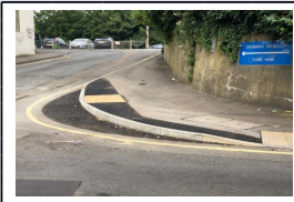
7th June - Carriageway widening for the diversion route ahead of the start of Phase 2
