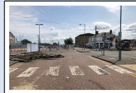
13th June - Area in front of the station hoarded off to the public
