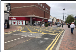
11th June - Yellow box junction installed in West Street/Station Street for the diversion route
