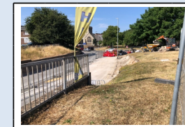
24th July - Excavation for the new retaining wall between Dover Street & Fountain Street
