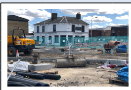
31st July - Formation of the roundabout in front of the car park entrance and Lang's Cocktail Bar
