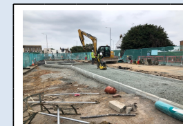
4th September - Construction of the bus stop/stand area in St. Michael's Road
