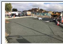
13th August - sub-base being installed to join new road layout to existing St. Michael's Road
