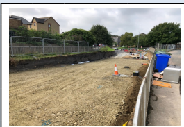
6th September - Material build up for the new carriageway level in Dover Street
