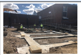
31st July - Foundations for the South West corner of the MSCP complete
