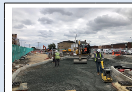
14th August - sub-base being installed at the exit to the new taxi rank area
