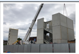
14th August - Continued assembly of the Western Stair Core and Lift Shaft
