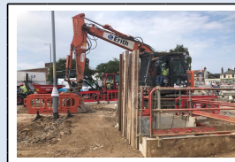
4th July - Sheet piling/trench boxes used to support the ground for deeper excavations
