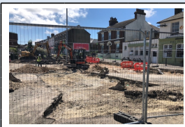
20th June - Excavation for the new crossing island at the end of Dover Street
