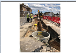
21st June - Installation of a new surface water manhole and pipework in front of the station
